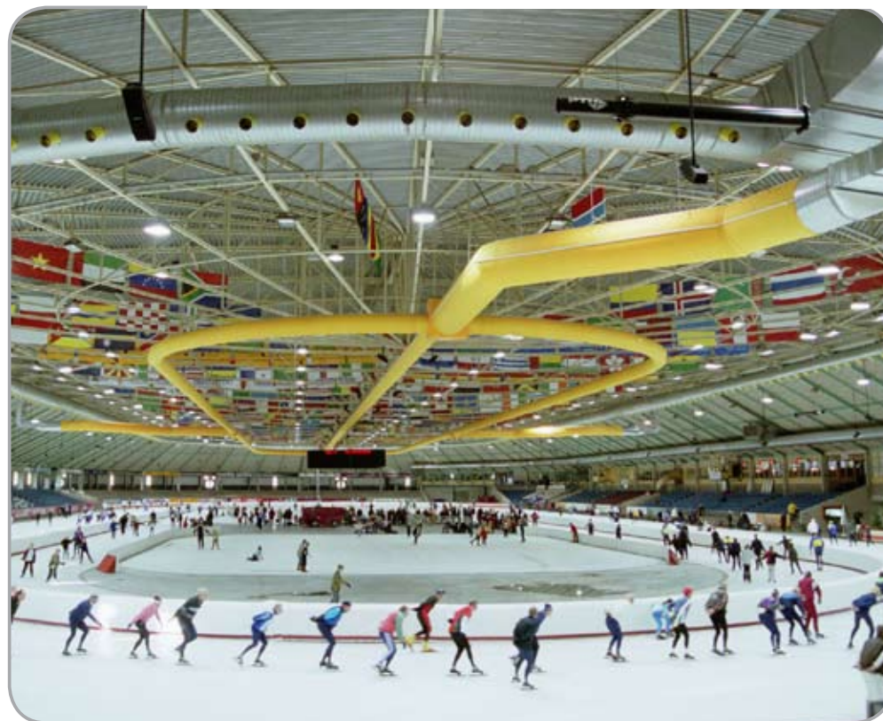
Thialf Heerenveen Ice Rink in the Netherlands fitted with yellow ventilation ducts
