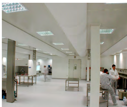
Clean room Alcon, Ireland
