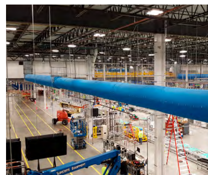
Daikin Texas Technology Park, USA
